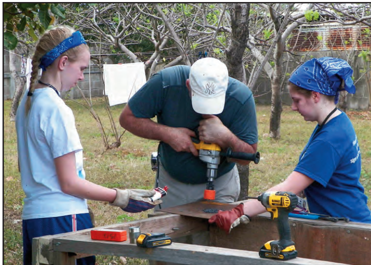
Sarah Rowen, left, waits for Allen Pellerin's instructions to add the oil as he drills a base for the cistern at Angels of Hope Orphanage in El Crucero, Nicaragua. Corinne White holds the base.
